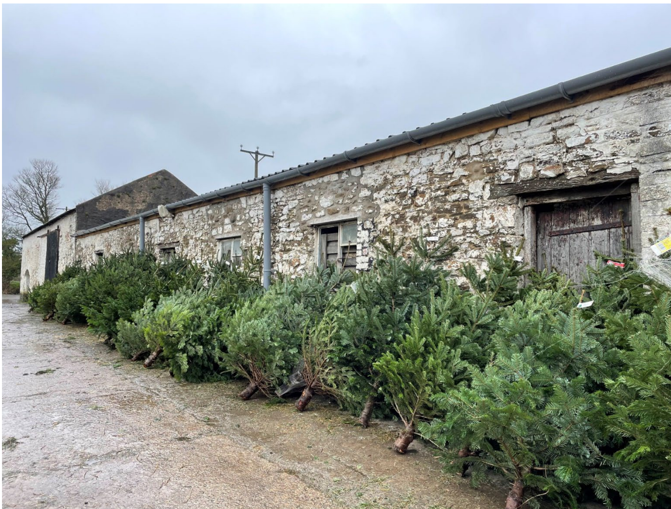
3. West-north-west facing elevation of single-storey range to the south-east of the farmhouse
