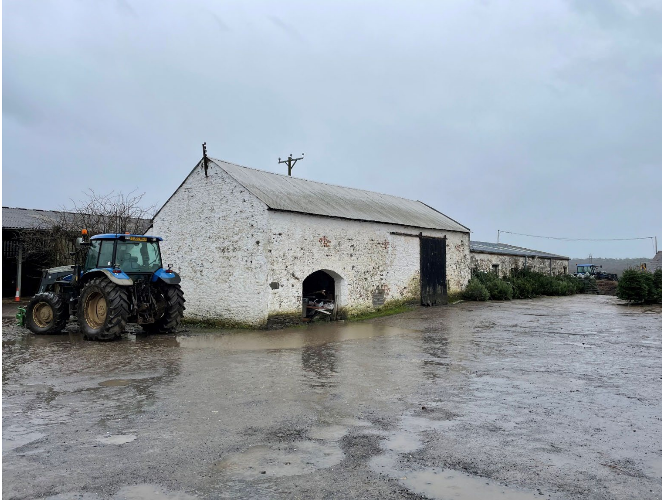
2. One-and-a-half storey barn and attached single storey range located to the south-east of the farmhouse
